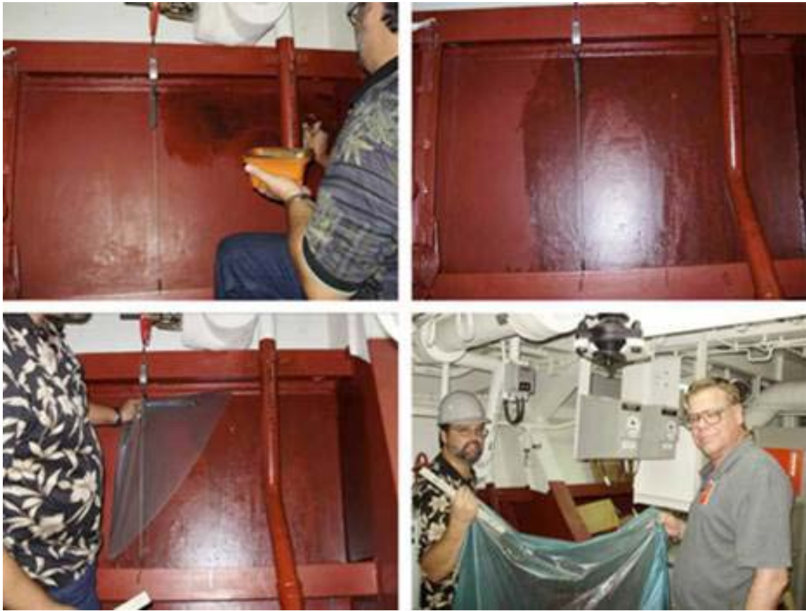
Figure 1. Use of polymer hydrogel for surface decontamination in ships. (upper left) Application with brush, (upper right) dried film in place, (lower left) peeling of dried film, and (lower right) sheet of dried film incorporating surface contaminants.
